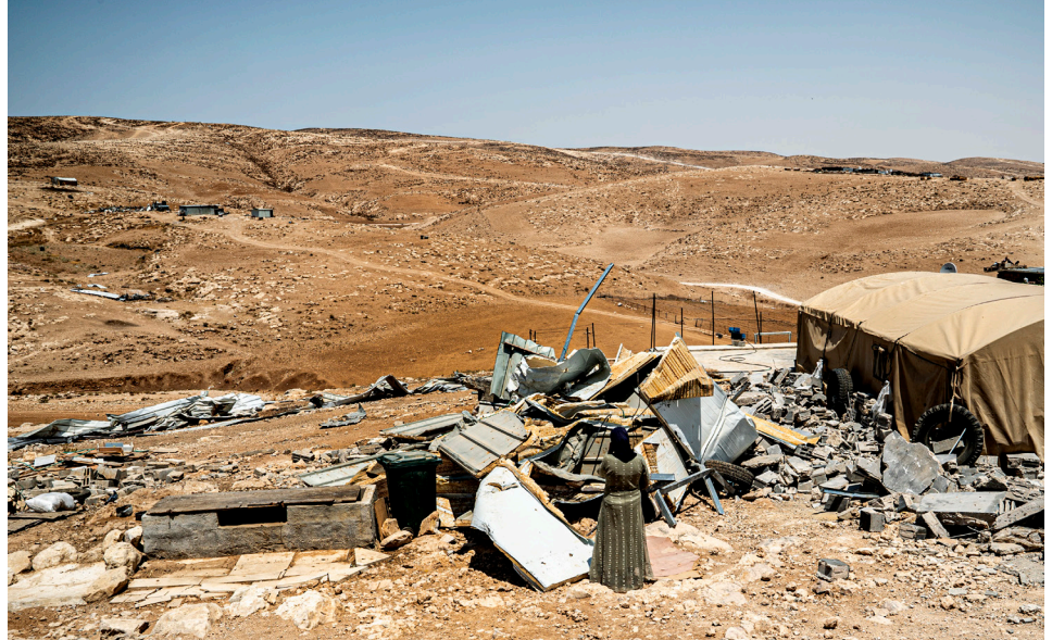
© JUAN CARLOS TOMASI Demolished shelter in Masafer Yatta, West Bank, Occupied Palestinian Territories.
